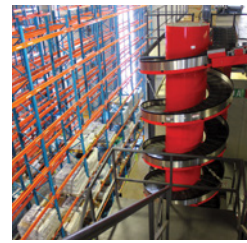
Warehouse Automation Systems
